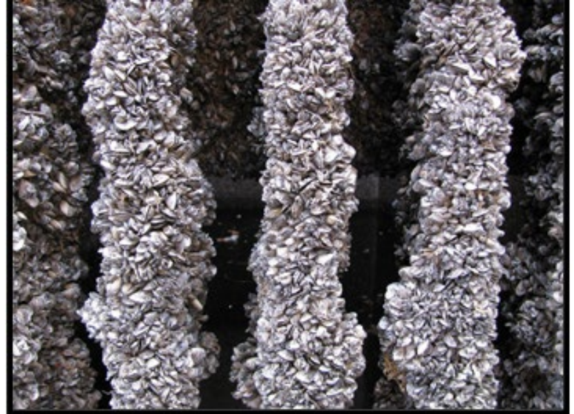
Trash Racks – Hoover Dam Circa 2010
