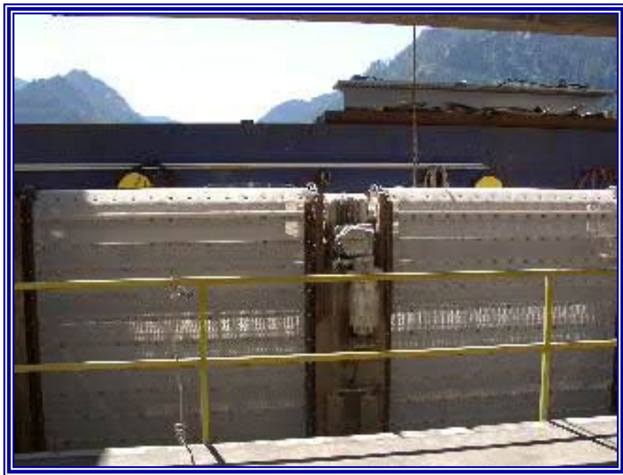
Travelling Fish Screens Bonneville Dam
