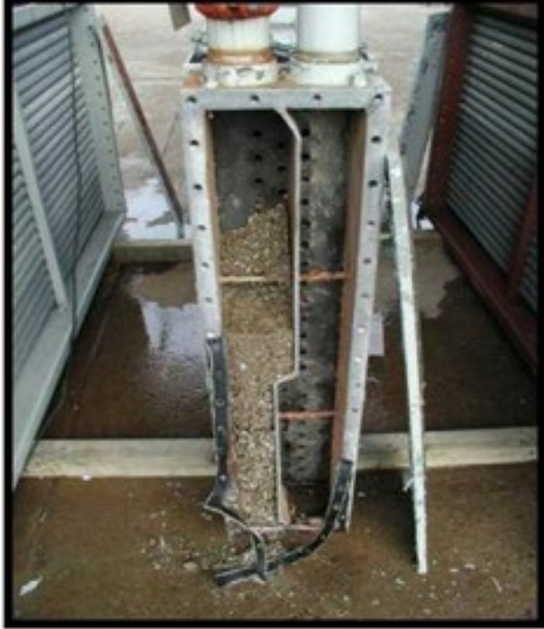
Cooler Unit w/Mussel Biofouling Ontario Hydro Early 1990's
